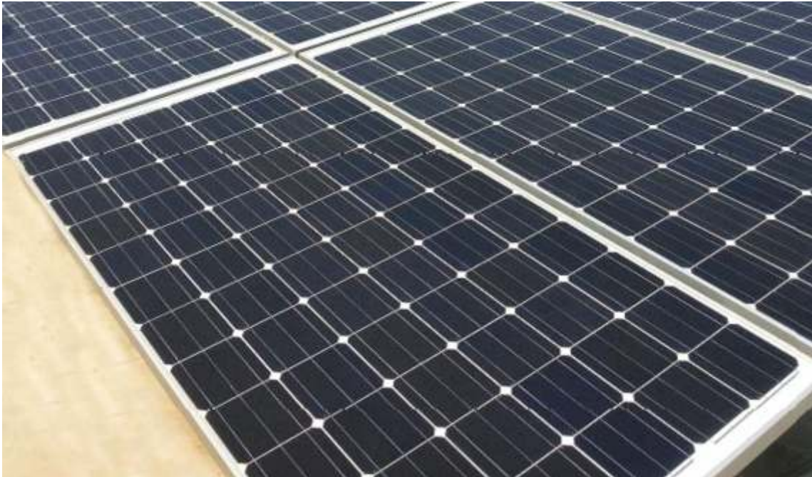
1st Solar Roof Top Project Synchronized with the Grid at Jubilee Hills, Hyderabad
